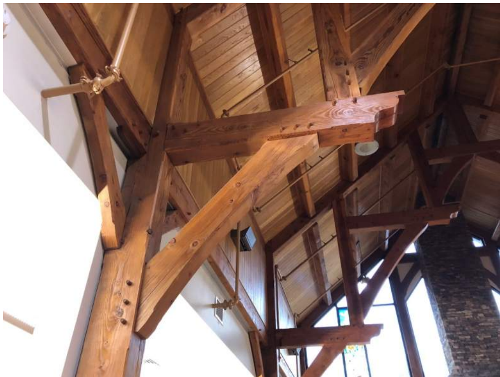
Photograph 12: Lower 'hammer' frame – slight downward rotation was observed.
