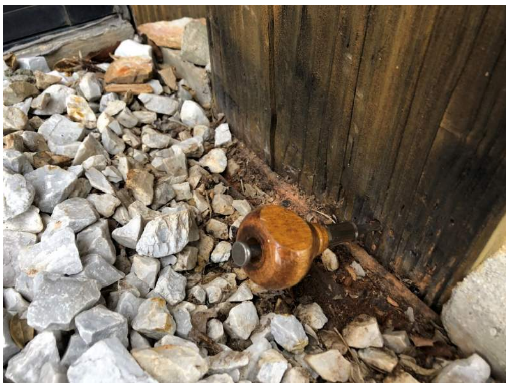
Photograph 9: Decay at base of timber column adjacent to main entry.
