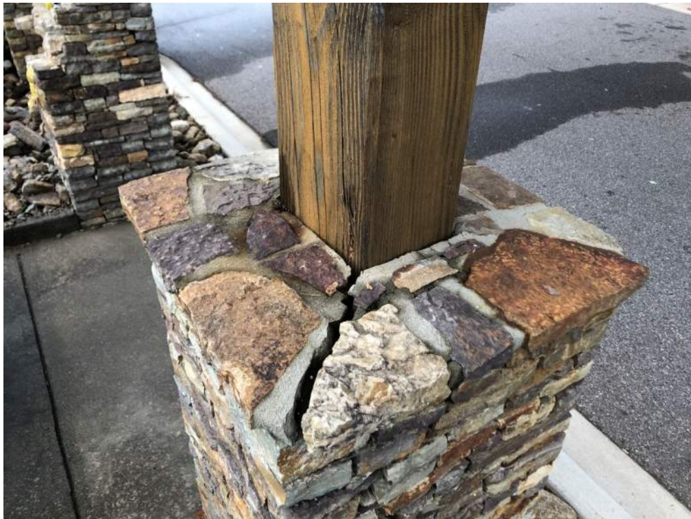
Photograph 4: Porte Cochere column with cracked stone cladding.
