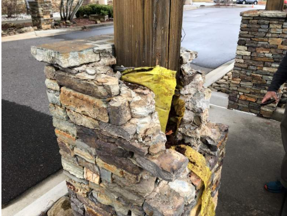
Photograph 3: Damaged column with stone cladding removed.
