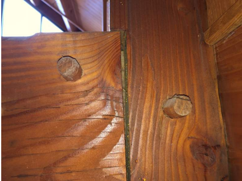
Photograph 13: Close up of joint at lower 'hammer' frame – some rotation was observed.
