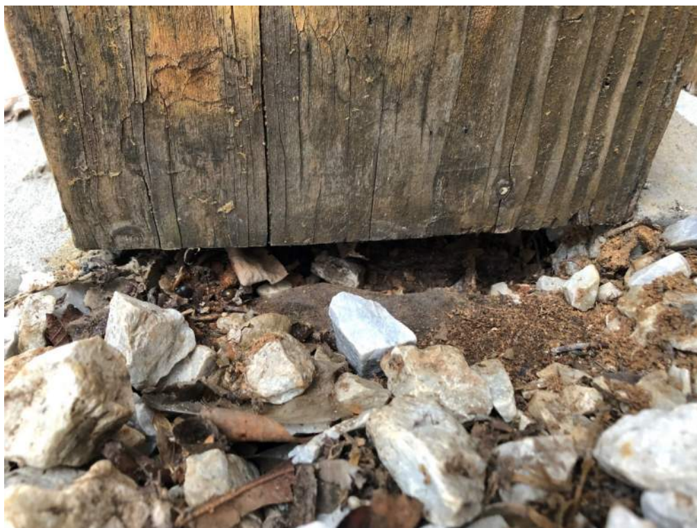
Photograph 10: Base of timber column adjacent to main entry in contact with soil and concrete.
