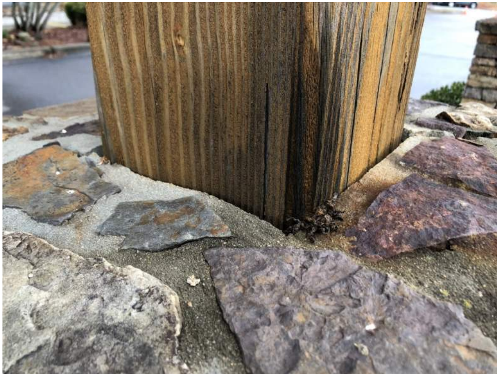
Photograph 2: Typical Porte Cochere column – note open joint allowing moisture intrusion.
