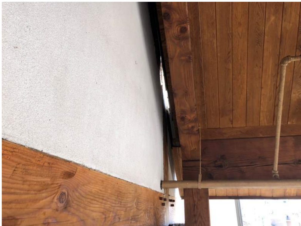
Photograph 6: Separation of connector roof from main building.
