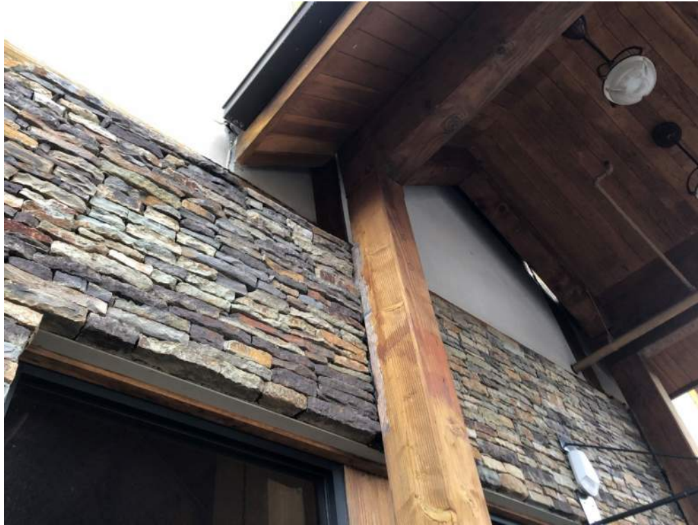
Photograph 5: Separation of connector roof from main building.
